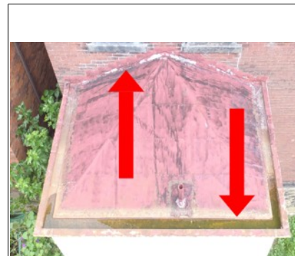
Poor flashing Gutters in need of cleaning
