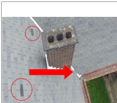
Missing tabs or shingles recommend repair or replacement.
