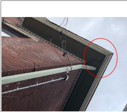
Entire soffit and trim in need of painting and repair
