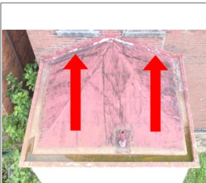
Flashing at roof edge and siding is in need of repair and sealing
