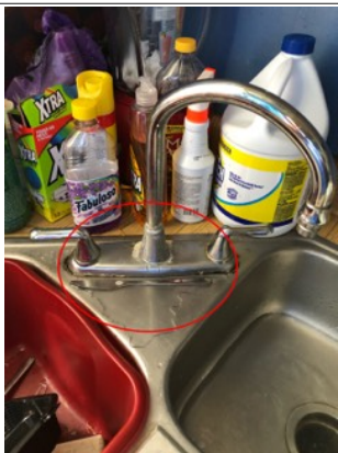
Faucet leaks at base
