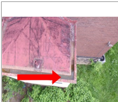
Gutters are in need of cleaning
