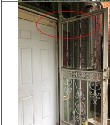
Front storm door doesn't have safety door closer
