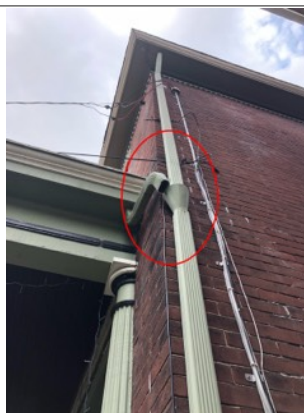
Downspout is not attached properly to other downspout for adequate drainage. This condition results in runoff puddling at foundation and contributing to water penetration in the basement
