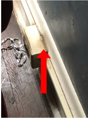
Owner shut off electric to entire upstairs, evidence of previous overheating and potential fire damage at outlet. Recommend electrician replace/repair and perform necessary safety checks before returning power to upstairs
